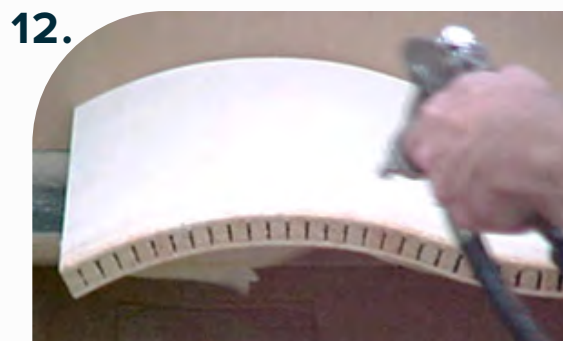
Apply adhesive to panel edge. Mask entire face to prevent glue overspray.
