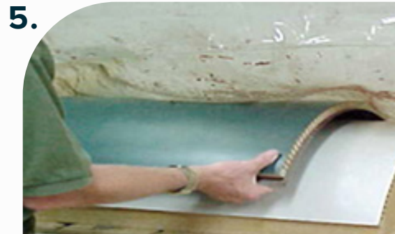
Place HPL face down on form. Then, place Kerfkore with glued rib side down onto HPL.
